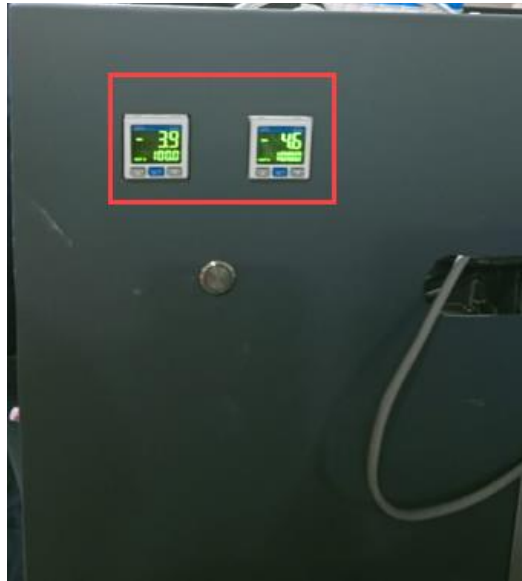
Figure 77: Negative Pressure Control Board
